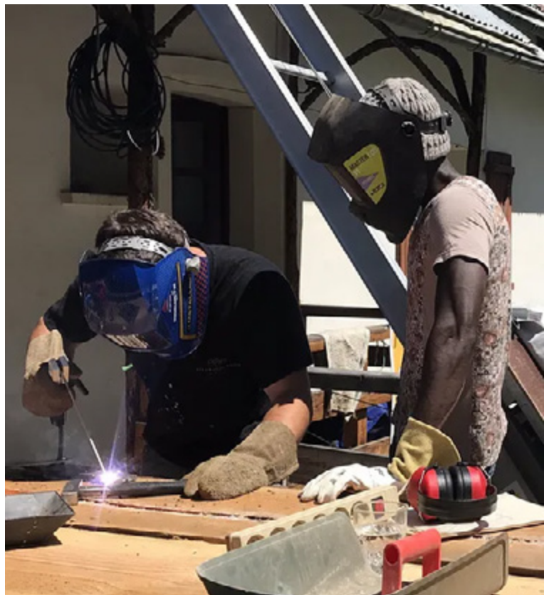
Right: Lamine, developing a vocation for the craft of welding, and Guillaume, professional welder©2020_EKO!
